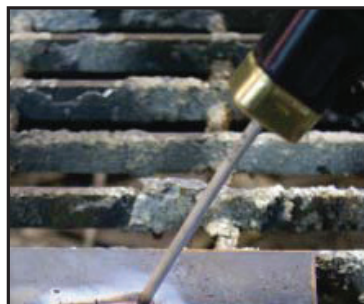
(7) To finish the weld, break the arc by quickly snapping the electrode away from the work piece.
