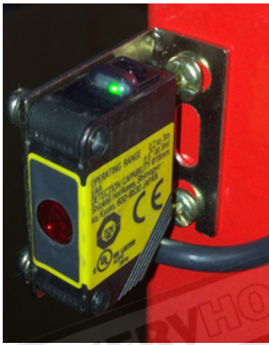
Power on but not aligned
